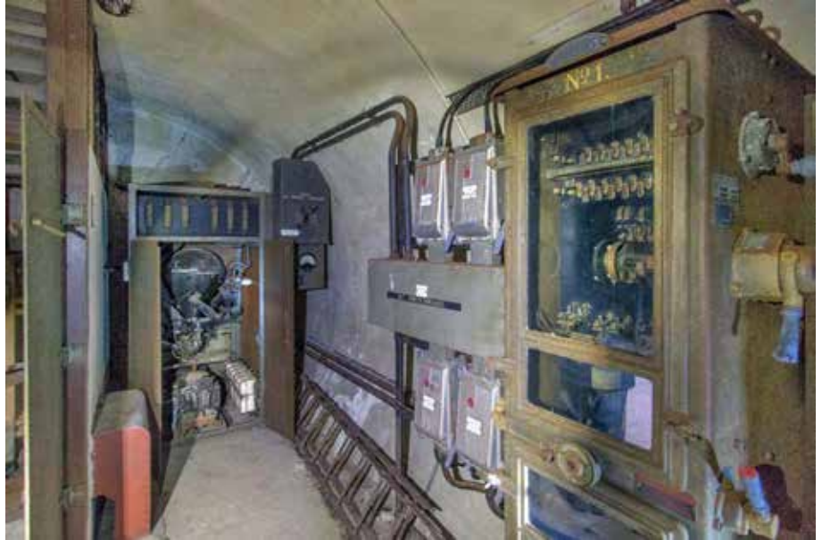
The most impressive feature of the plant room is the mercury vapour rectifier which is original and was still in use until the lift was taken out of use. The mains transformer that fed the rectifier is in the cabinet to the left. The cabinets on the right contain rheostats for controlling the speed of the fan
